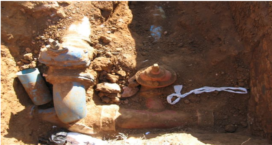
Photo 1.1 – Typical example of an unknown connection
